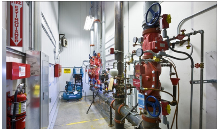
Coastal Pacific Food Distributors installed variable frequency drives (VFDs) on all dry motors and compressors in their new freezer
