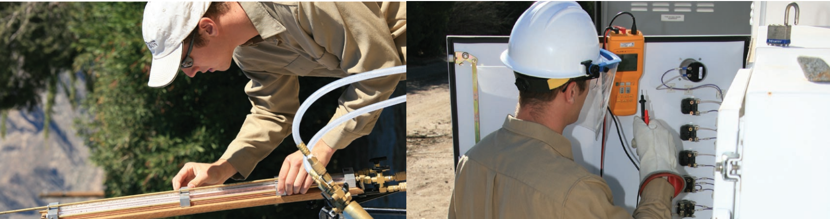
Express Solutions, AP-I and Free Pump Testing from SCE Help The City of San Bernardino Municipal Water Department Maintain Quality and Save Money
