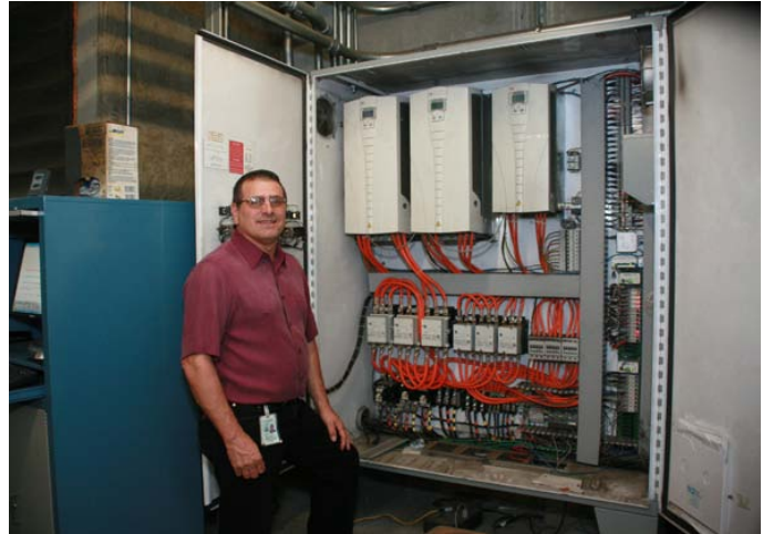
Bill Ellena, corporate maintenance manager at Coastal Pacific Food Distributors, said that in 12 months on the Critical Peak Pricing rate, "I've used more electricity, but I've saved about $60,000 (in direct savings and avoided costs)."
