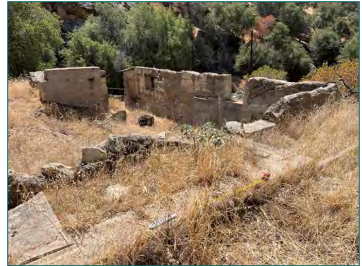
Camp 4 Locus A2, overview of remains of Dam Tender's Cottage, view east
