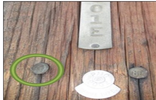
Figure 15.4: Nail Below Pole Tag – Length 70 ft
