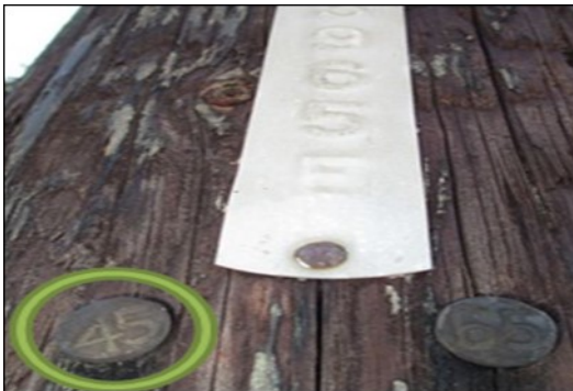
Figure 15.3: Nail Below Pole Tag – Length 45 ft
