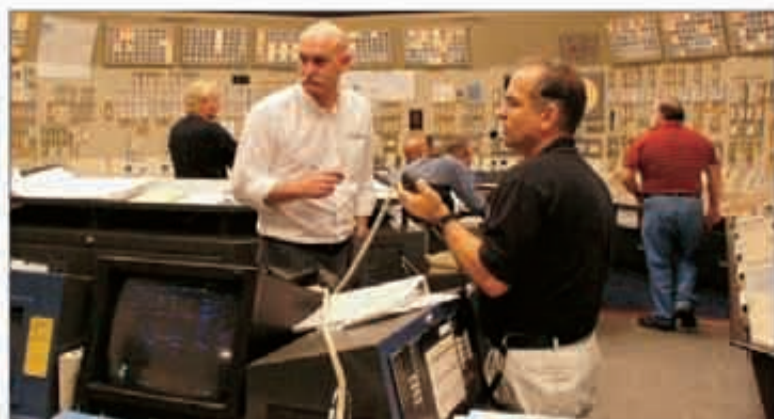
State-of-the-art controls at San Onofre constantly monitor plant conditions to ensure optimum safety for the public and plant personnel.
