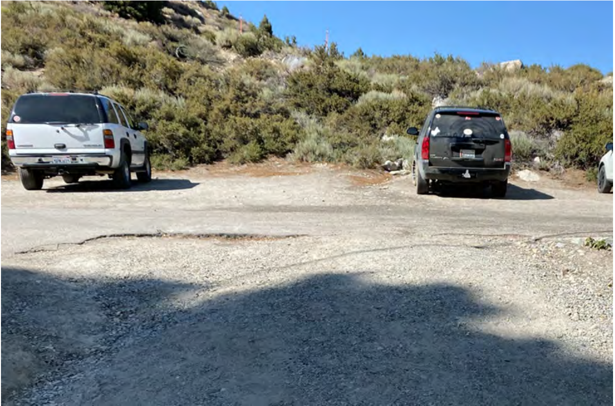
Photo 90 Eroded Edges of Paved Surfaces
