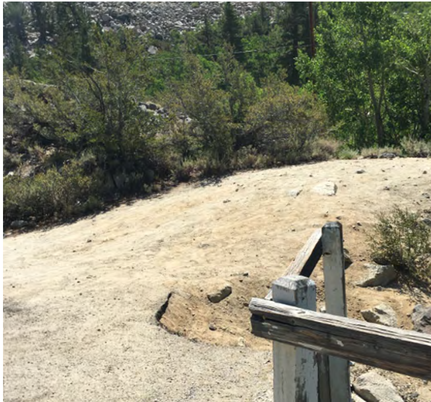
Photo 11 Eroding Edge of Roadway
