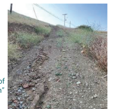
Right: Example of road in "Fair Condition"
