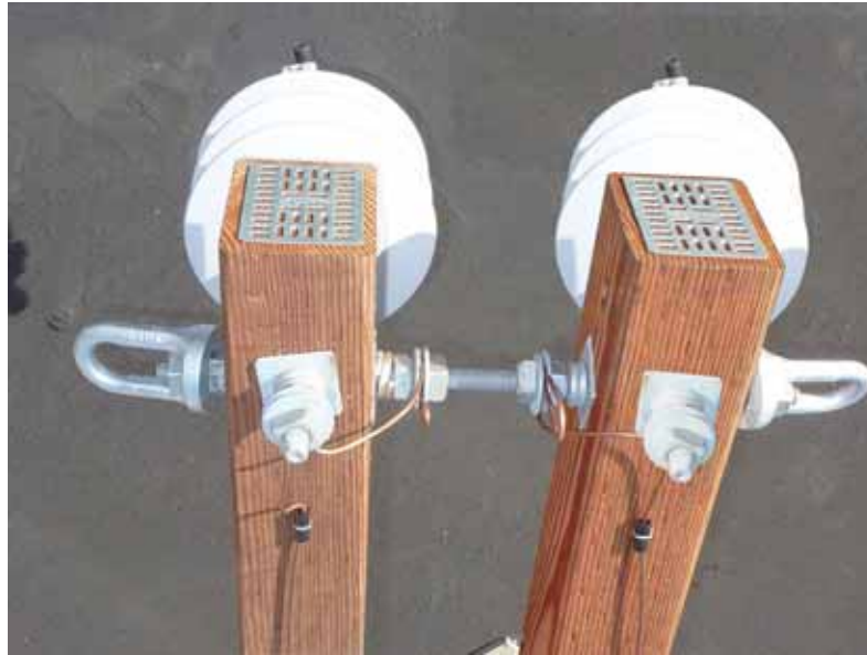
Figure DC 612-8: Typical Spring Washer Hardware Assembly for Double Crossarm and Bonding
