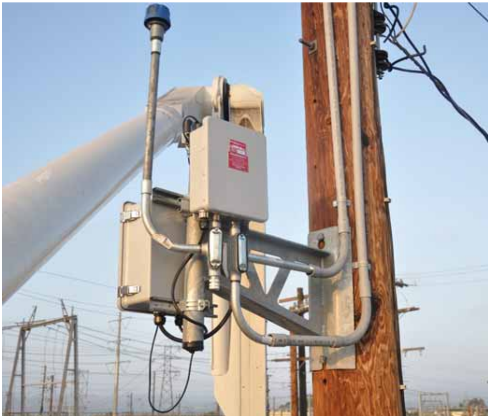
Figure SL 601–4: Typical Installation of FAA Lights on Distribution Poles (Control Panels and Photocell)
