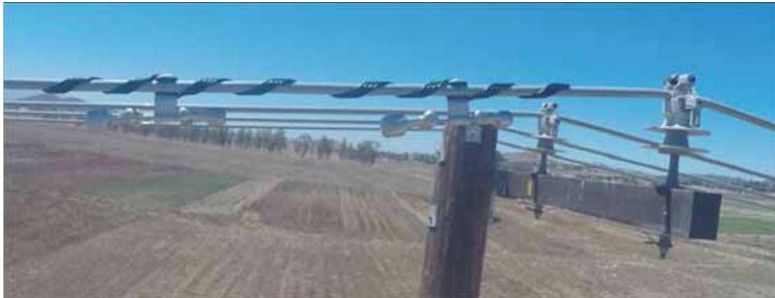
Figure CC 190–13: Installed Spiral Rod Stockbridge Damper
