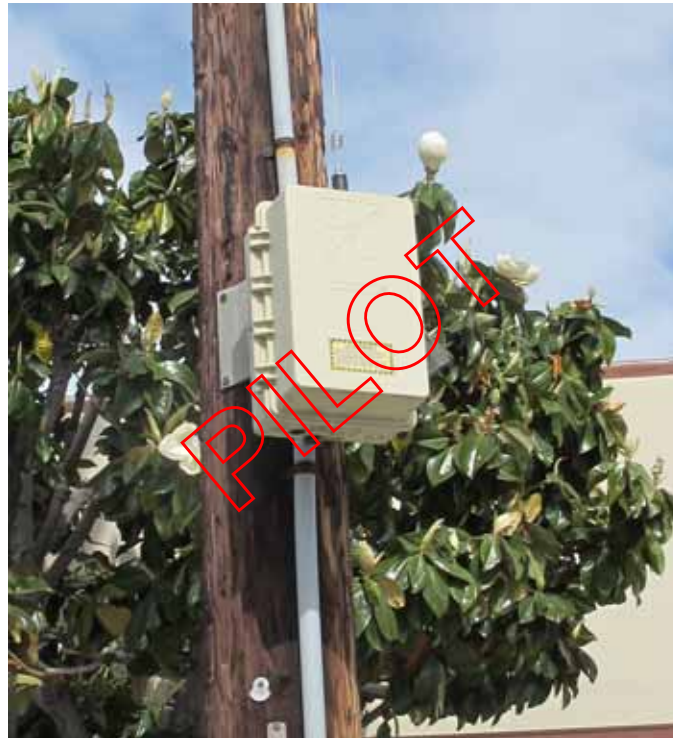
Figure IGP 110P–1: Capacitor Controller Manufacturer Radio
