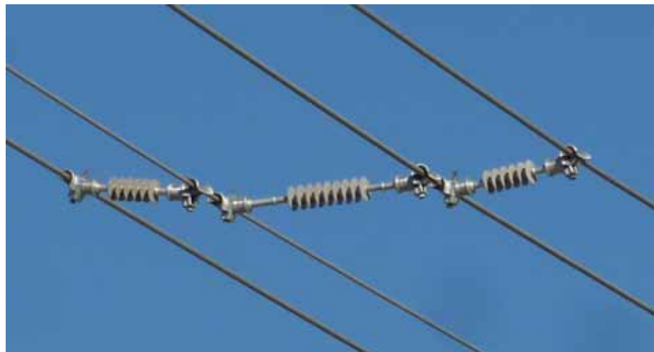
Figure 450-1: Insulated Overhead Wire Spacers Installed on a Horizontal 4-Conductor System
