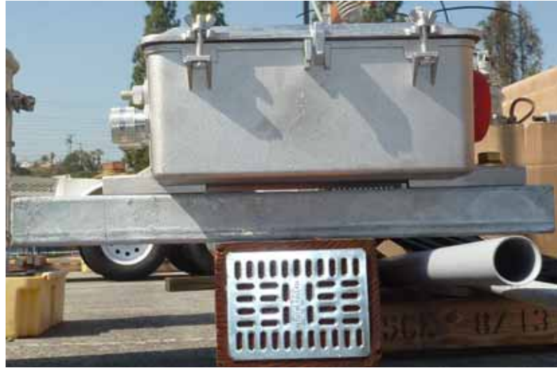
Figure SL 500–3: RCOC Relay Installation on Unistrut
