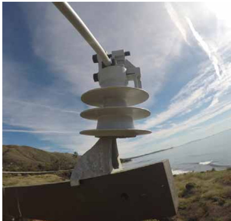
Figure CC 150–1: Covered Conductor on Vice-Top, Nylon Insert Insulator
