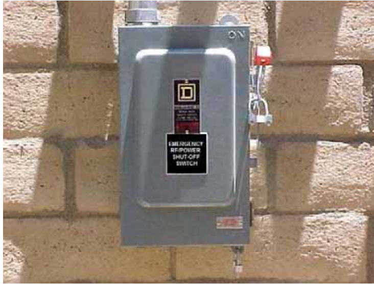
Figure DC 222–5: Emergency RF/Power Shut-Off Switch
