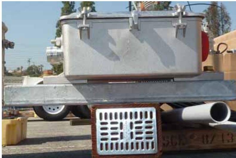
Figure SL 505-2: RCOC Relay Installation on Unistrut
