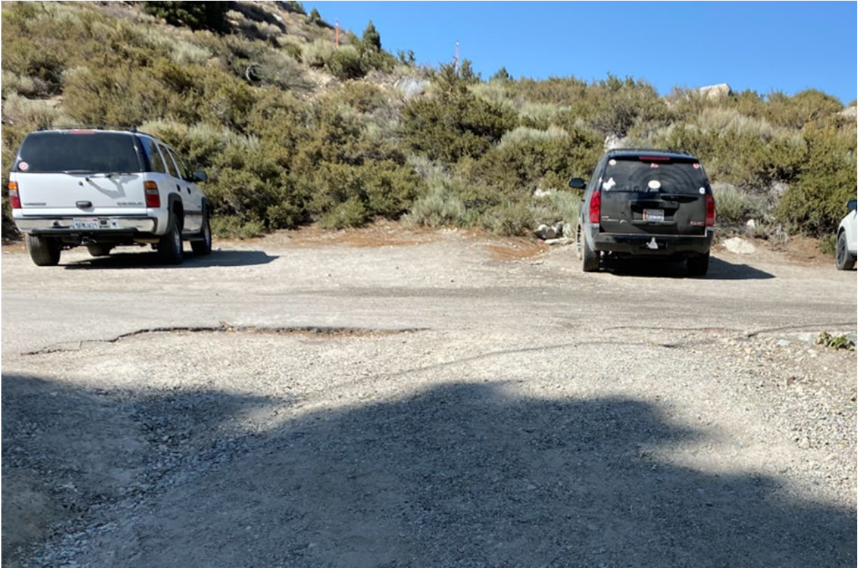
Photo 90 Eroded Edges of Paved Surfaces
