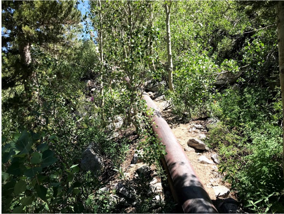
Photo 55 Green Creek Diversion Pipeline Adjacent to Rainbow Pack Station Trail
