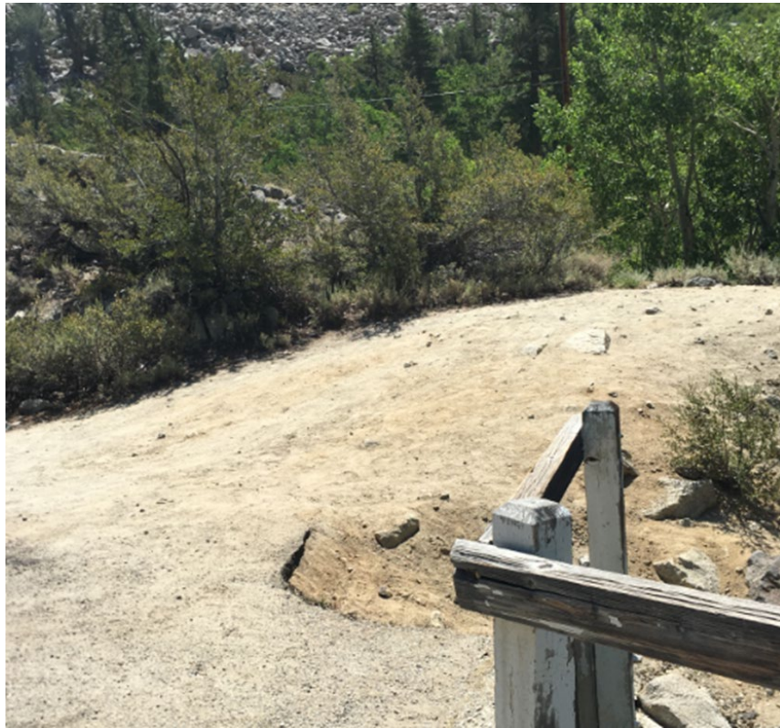
Photo 11 Eroding Edge of Roadway
