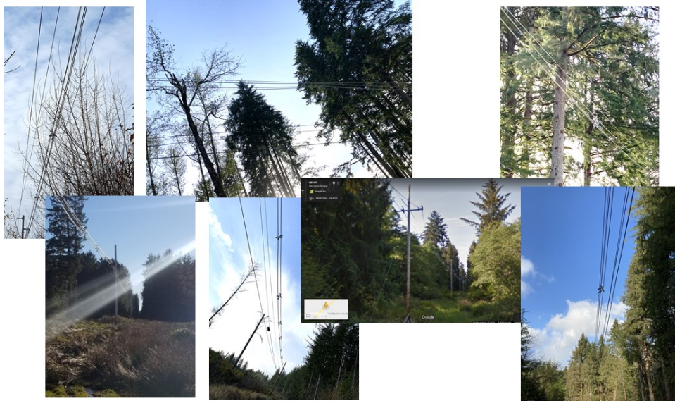
Figure CC-5 PacifiCorp Covered Conductor Effectiveness Examples
