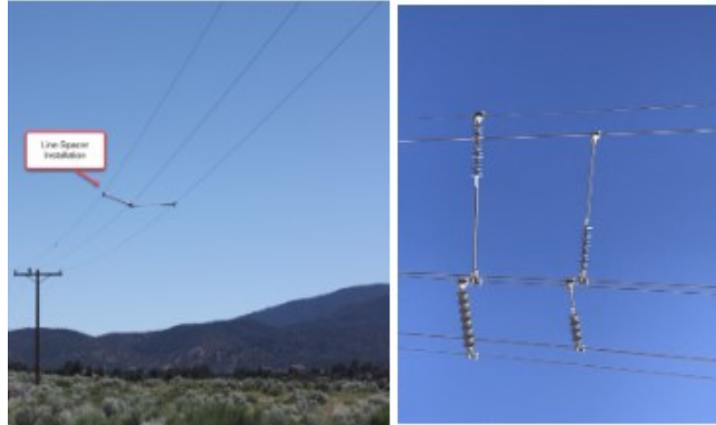
Figure SCE 8-08 - A Line Spacer Installed on a Long Span to Mitigate Wire-to-Wire Contact (Left), Close Up Line Spacer View (Right)
