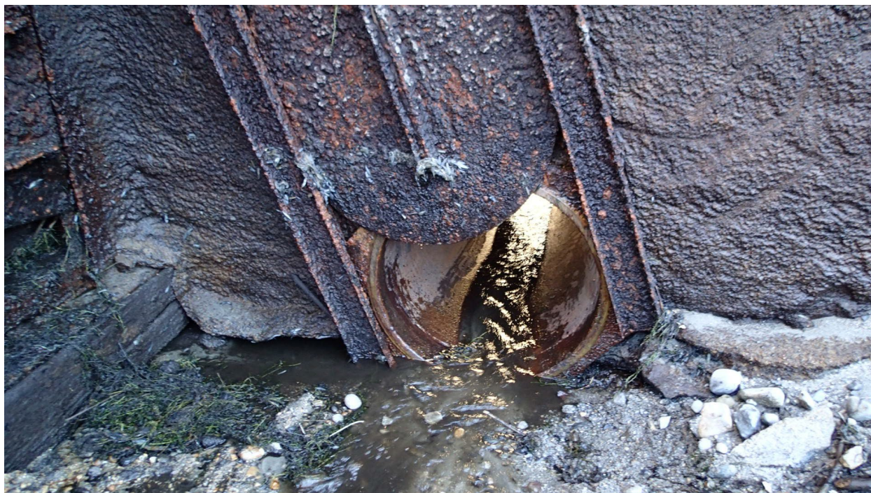
Figure 4.1-1 Intake No. 5 Low-Level Outlet Slide Gate.
